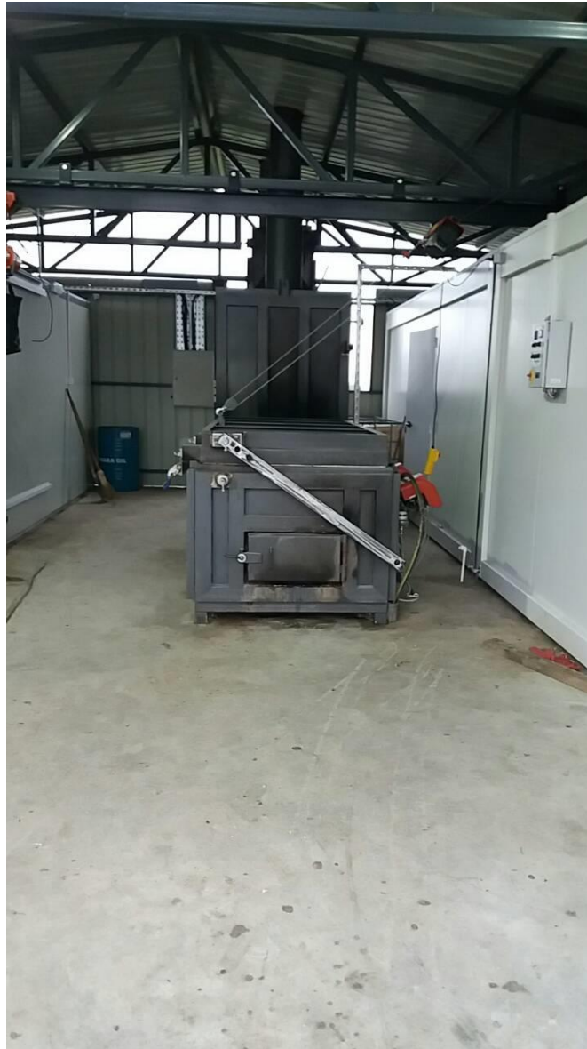
Fig. 1. Incinerator INCINER8 Model I8-250, on the right side there is a sanitary and office container, and on the left side there is a refrigerator of container type.
