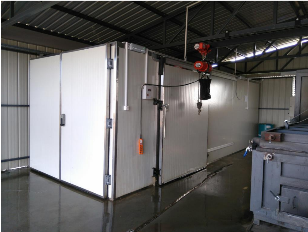
Fig. 2. Cold store for temporary storage of animal corpses and remains with a crane that transfers animal material from the cold store to the incinerator.
