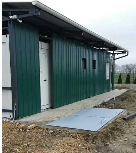
Fig. 5 The position of the underground tank and place of the fuel overflow.
