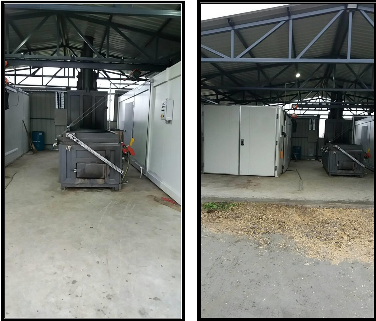
Fig. 3 and 4 Steel canopy with equipment for incineration of animal by-products, carcasses and materials
